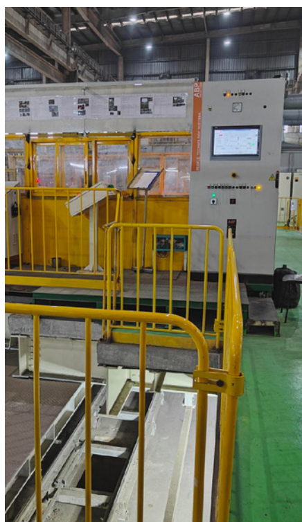
All furnaces and systems were installed on time.
